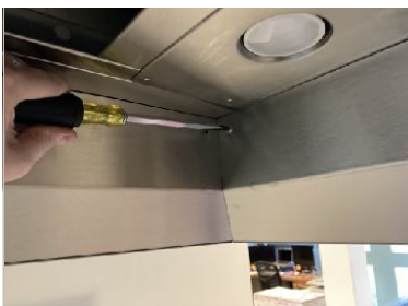
31. Once the side trim panels are secured, carefully slide in and rotate the front trim panel into place between each side trim panel. Be careful not to scrape or mar the trim surface. Then install the remaining trim mounting screws.
