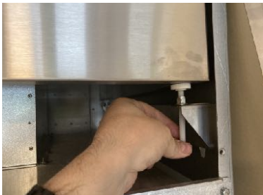
25. Install and raise the duct cover against the ceiling/soffit surface and if clearance allows, secure with appropriate screws into place.
