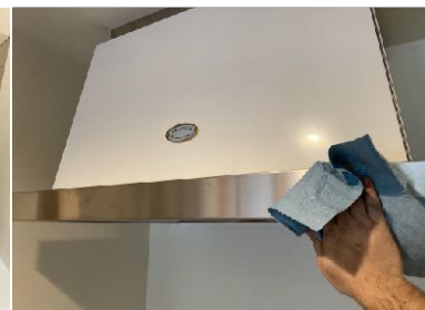
33. Test hood functions and clean unit with suggested cleaners. Install is now complete.
